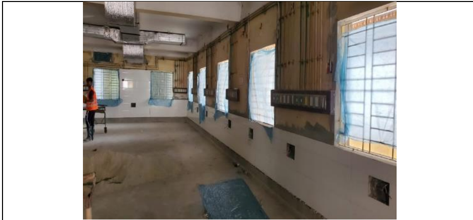
Windows are Covered at ICU and CCU Construction, Khulna Medical College Hospital
