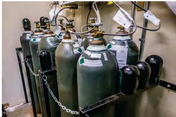
Figure: Cylinder storage with protective chain
