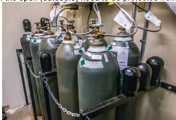
Figure: Cylinder storage with protective chain
