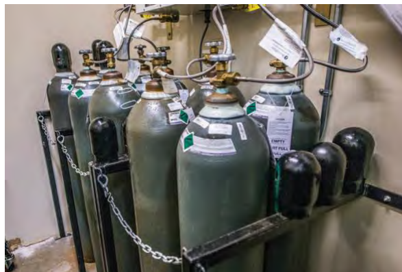
Figure: Cylinder storage with protective chain
