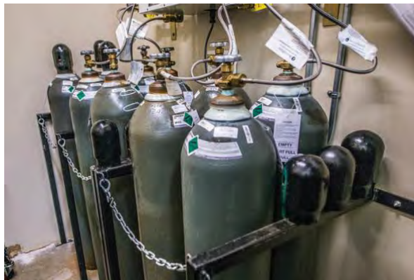
Figure: Cylinder storage with protective chain
