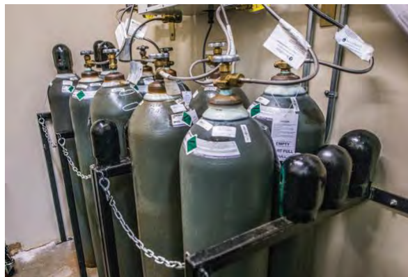
Figure: Cylinder storage with protective chain
