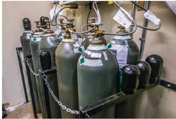
Figure: Cylinder storage with protective chain
